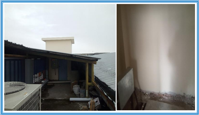
Rumah water dump lift, lt. rooftop
