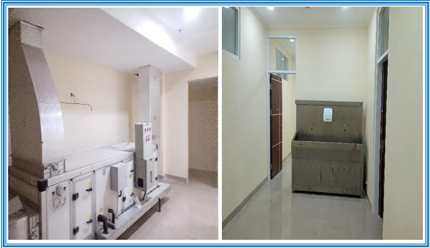
Area Ruang AHU &.Bak scrub station Lt. 03
