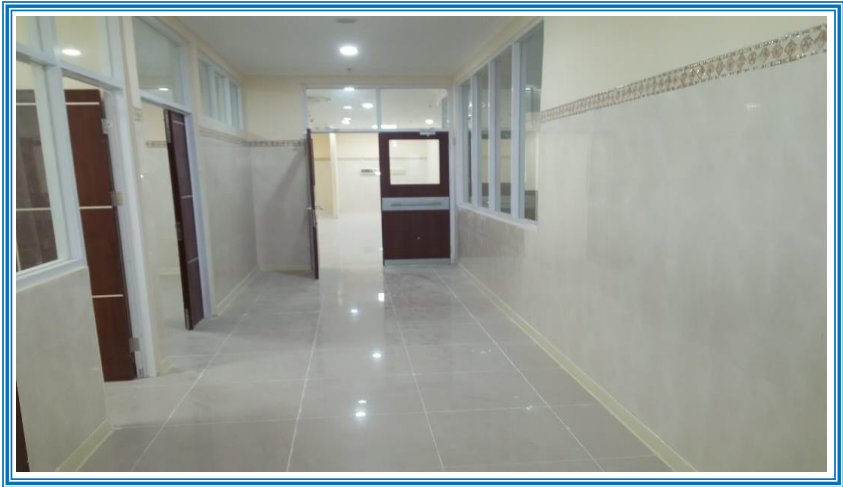
Air lock room Inst. ICCU lt. 03
